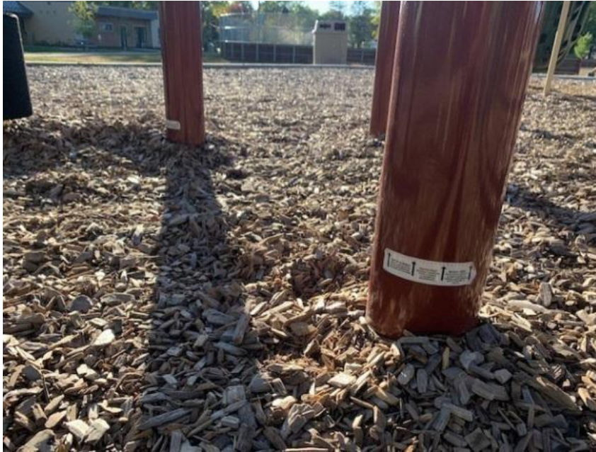
These wood chips are too low; they are supposed to be up to the white tag.
